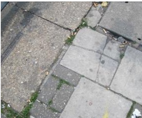
Poor quality public realm visually detracts from the area.
